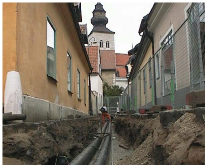
Figure 45: Installation of a district heating system below the streets of Visby’s historic city centre, a World Heritage Site (Image © GEAB)
